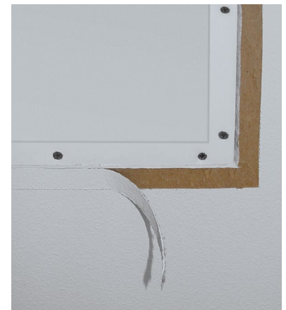
On a finished wall, create a space for the nylon mesh tape and mud by stripping back about 1" of the wallboard paper.
